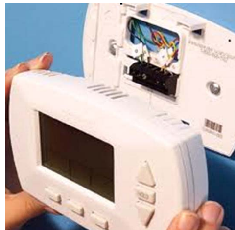
Install a Programmable Thermostat
